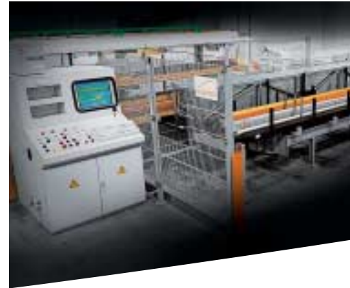
Example: Longitudinal rotary station with four cassette locations and minimized cassette change times.
