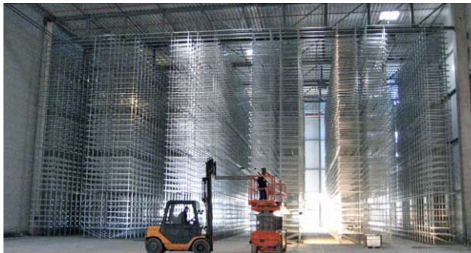
The automatic small parts storage system follows the "goods to picker" principle
